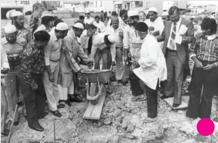
Suliman Bhikoo lays the foundation stone for the Al-Masjid Al Jamie, 30 March 1979.
